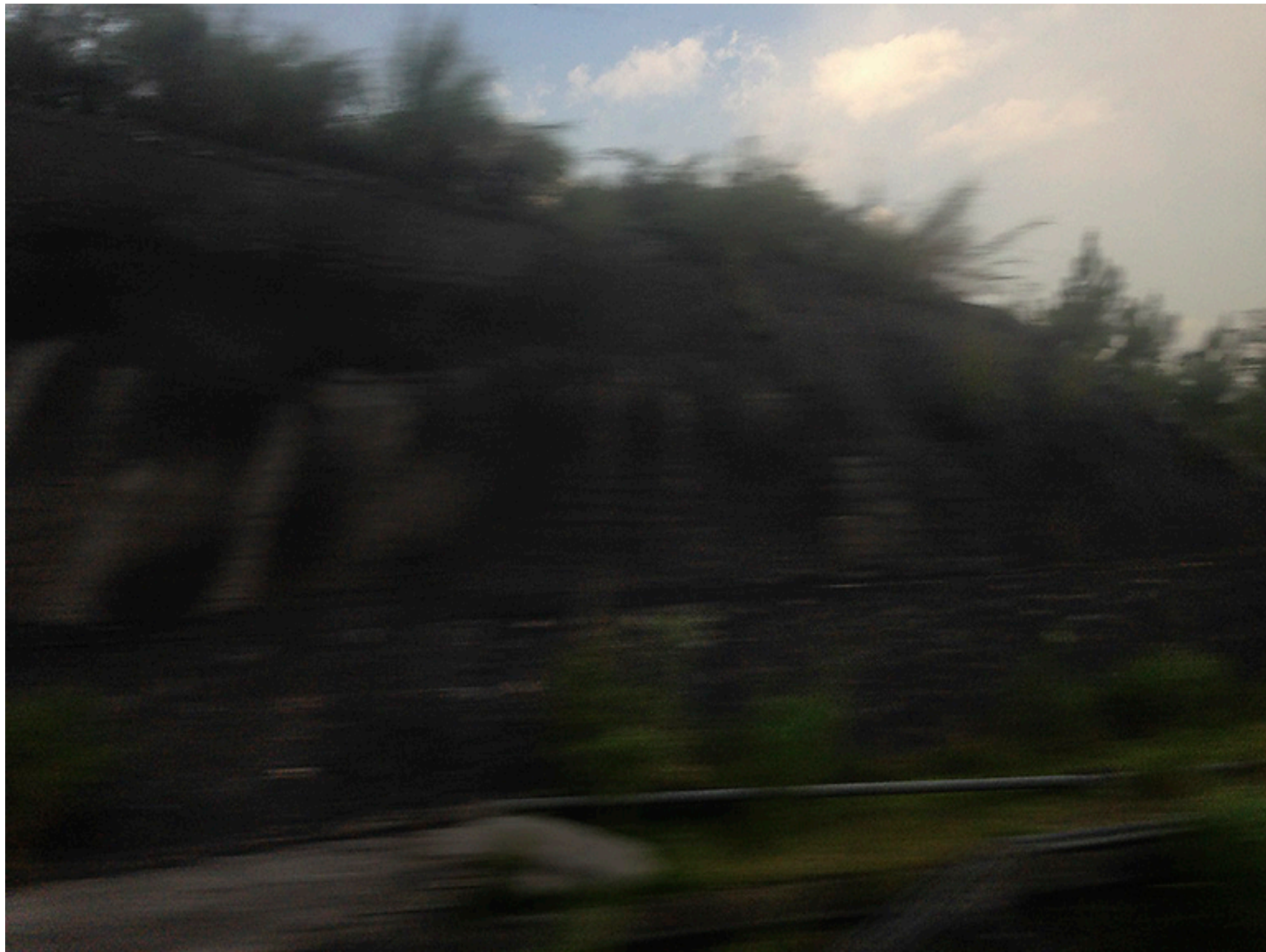
在挡土墙前的动态物体 Moving Object in front of the Retaining Wall 24x18cm
